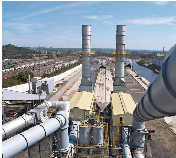
Dedusting system at Carionx, Belgium
