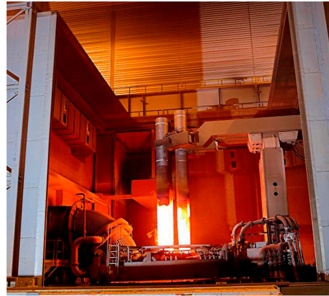
Noise protection doghouse at Carinox, Belgium
