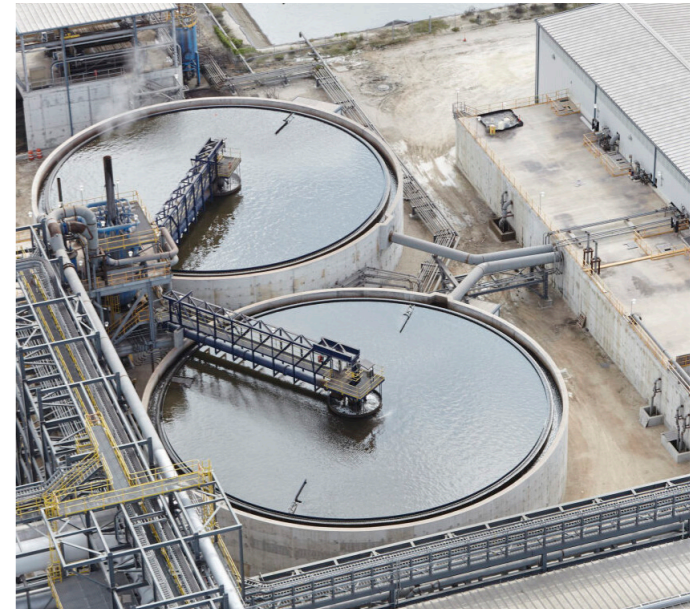
Water treatment system at ArcelorMittal, Texas
